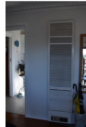
Gas wall furnace/heater (INT20)
