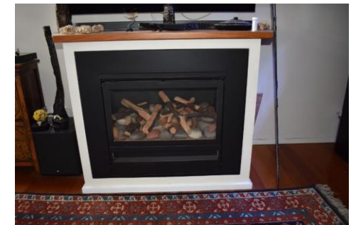
Gas room heater (INT11)
