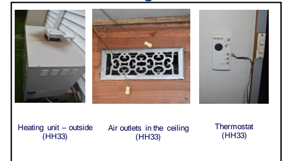
Ducted forced air heating system – through floor
